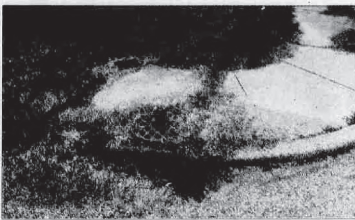
A storm drain sits lower than a sidewalk along Covert Avenue, which causes the street to flood when it rains heavily.
