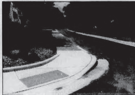
New sidewalks were laid in the Presidents neighborhood along Ravenswood Drive as part of a sewer project on the southeast side of Evansville.
